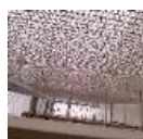
Metal Fabric Tensile Structure
