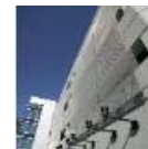
Exterior Metal Fabric Panels
